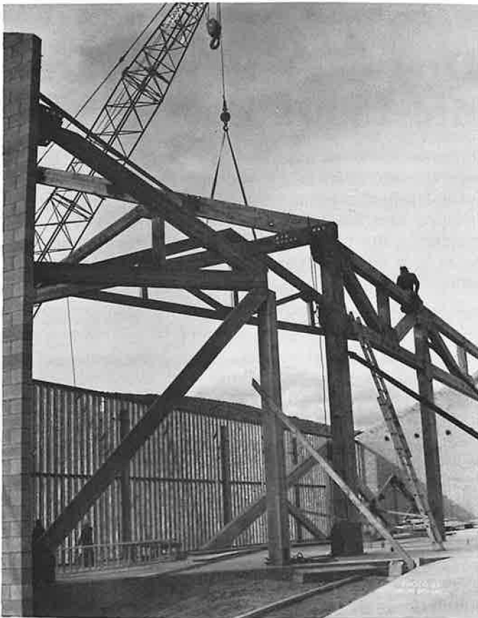
Daun Bohall photo illustrates the setting of roof trusses on the new Interpretive Center at the Nevada State Railroad Museum on Oct. 16, 1987.
