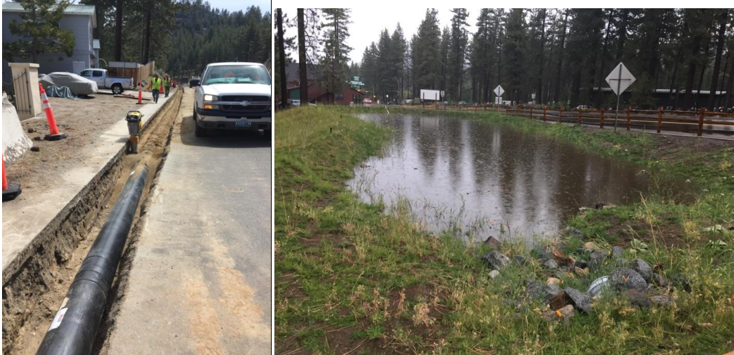
Zephyr Cove GID Water Quality Improvement Project: Left, installation of storm drain, Right, Newly constructed basin collecting runoff.
