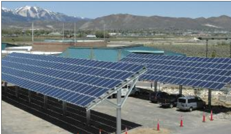
Solar panels at three Nevada Guard facilities serve as one of the state's alternative sources for energy.
