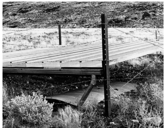
FIGURE 27. Fiberglass cisterns and all steel apron construction provide relatively maintenance-free guzzler installations in Nevada. (Photo by author.)
