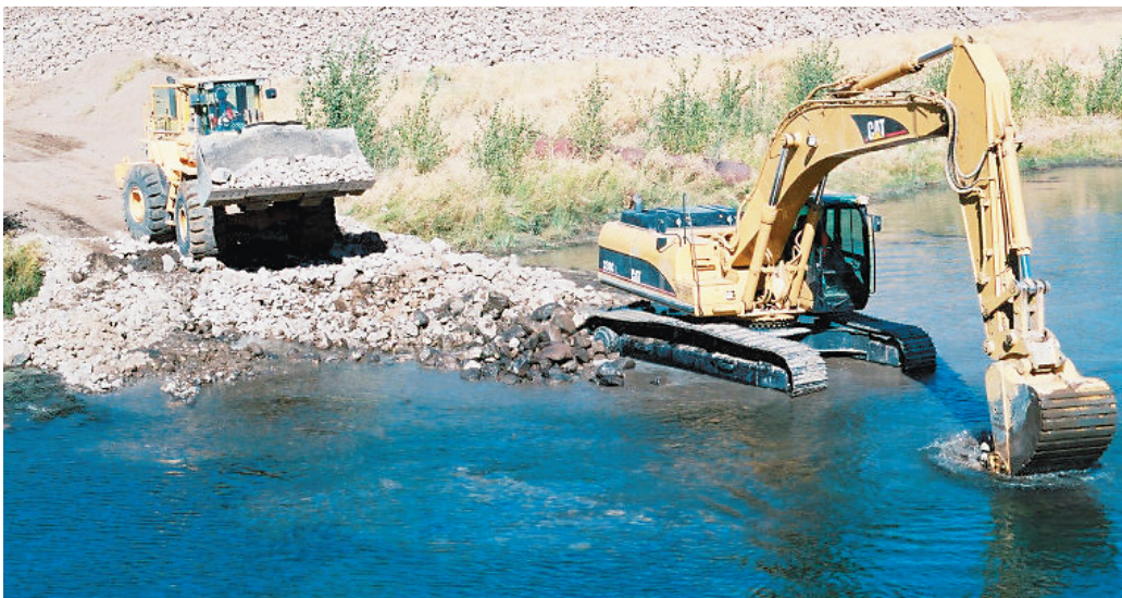
Truckee River restoration efforts are ongoing at The Nature Conservancy's McCarran Ranch.
