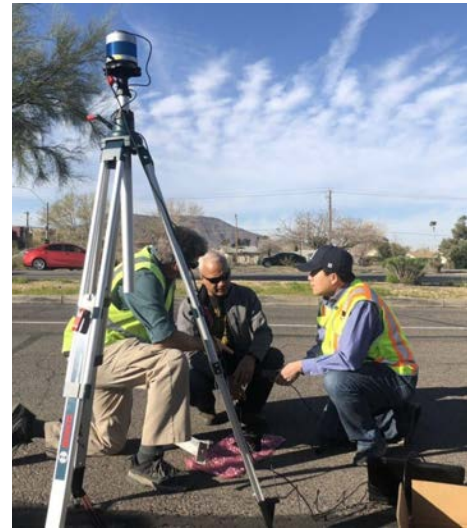
Hao Xu (right) works with engineers from RTC of Southern Nevada and the City of Henderson to set up a roadside LiDAR sensor. Photo taken prior to the COVID-19 pandemic.
