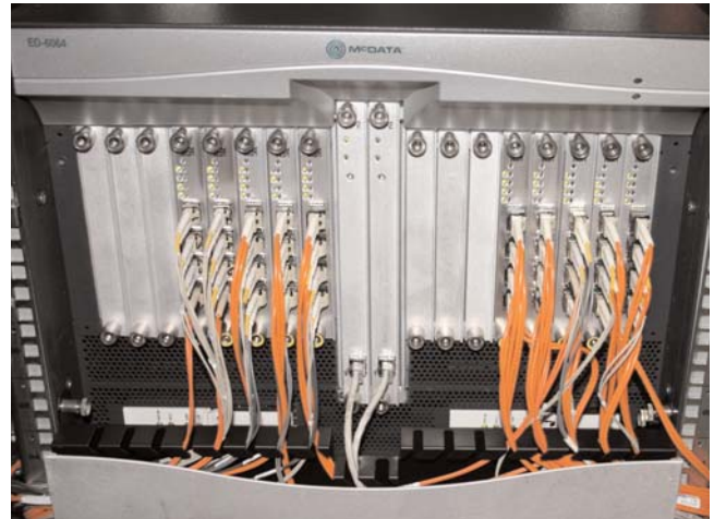
Fiber Optic Network Switch
