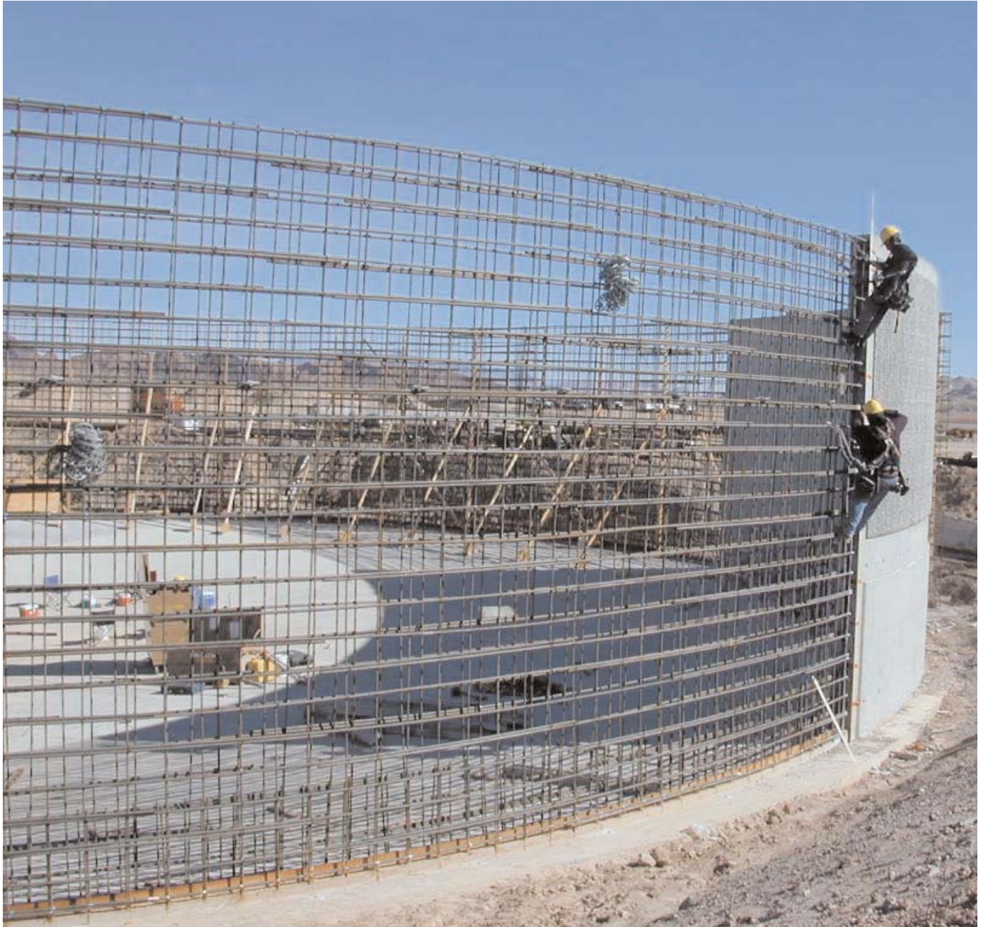
Flow equalization basin walls
