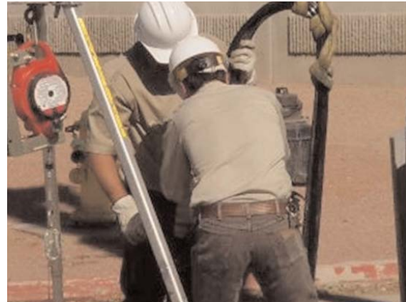
Maintenance of Utility System
