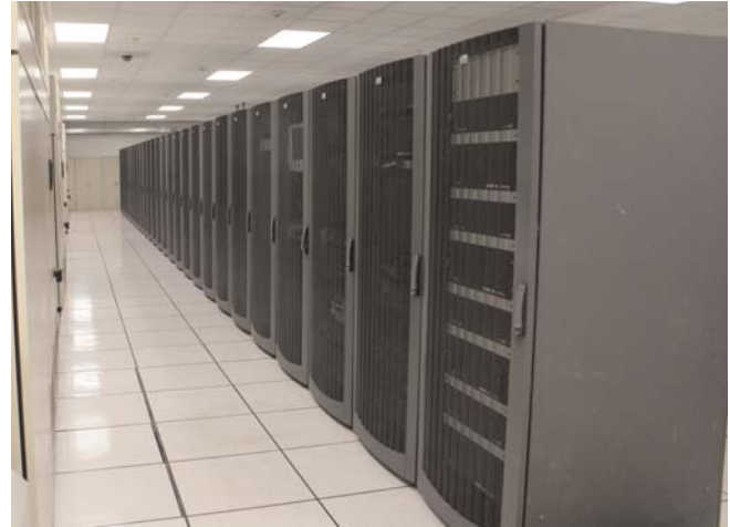
Server Room in City Hall Expansion
