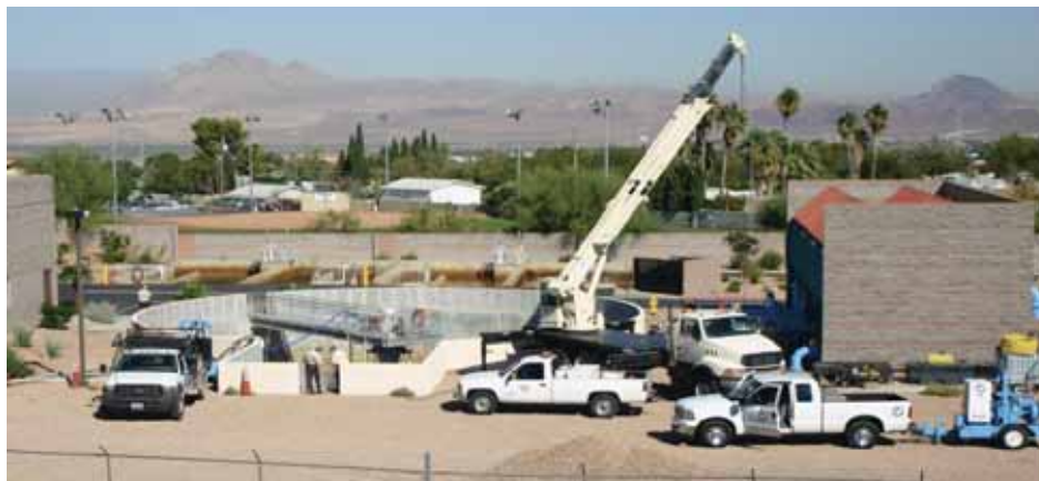
Backflow Recover Basin Maintenance
