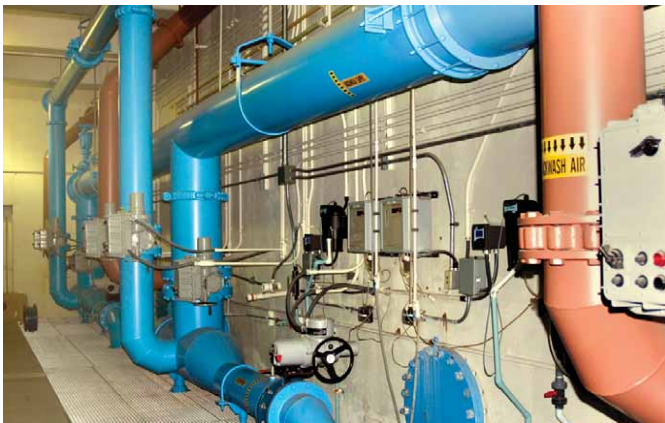
Water Treatment Facility
