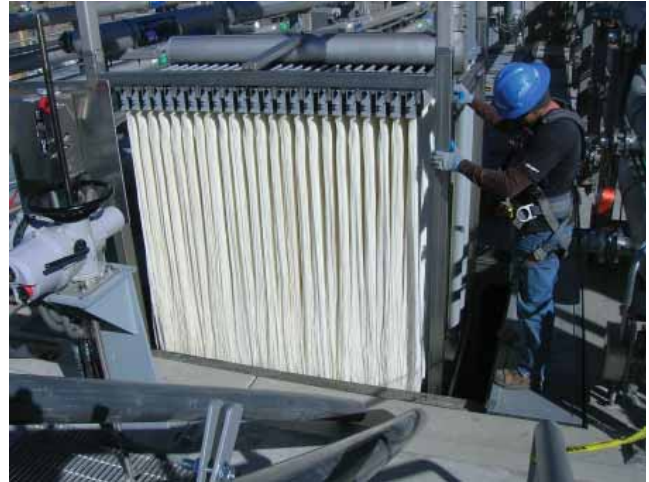
Membrane Filtration Installation
