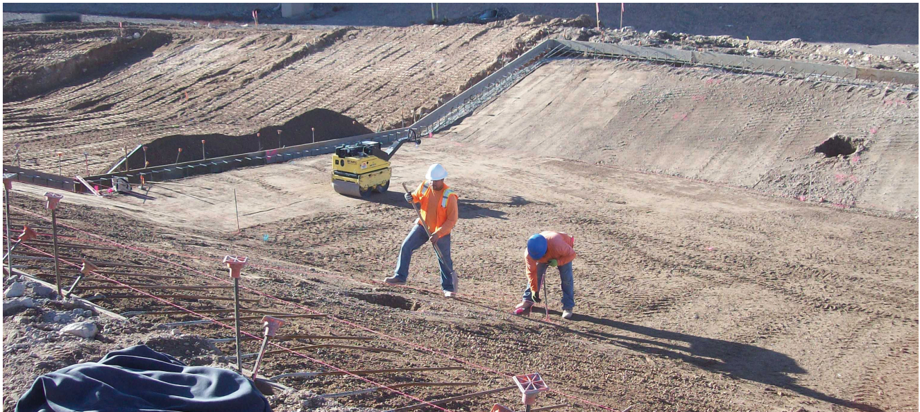
Pioneer Detention Basin Inflow Channel
