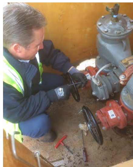
Backflow Prevention Assemblies – protecting our system
