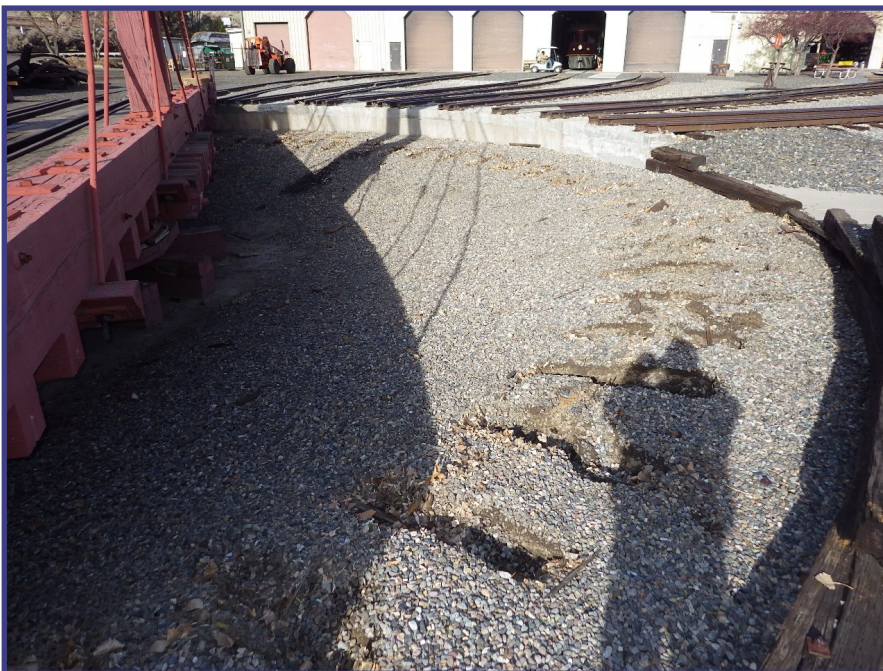
The outer ring rail was removed due to the damaged caused by the Jaguar. (NSRM photo)
