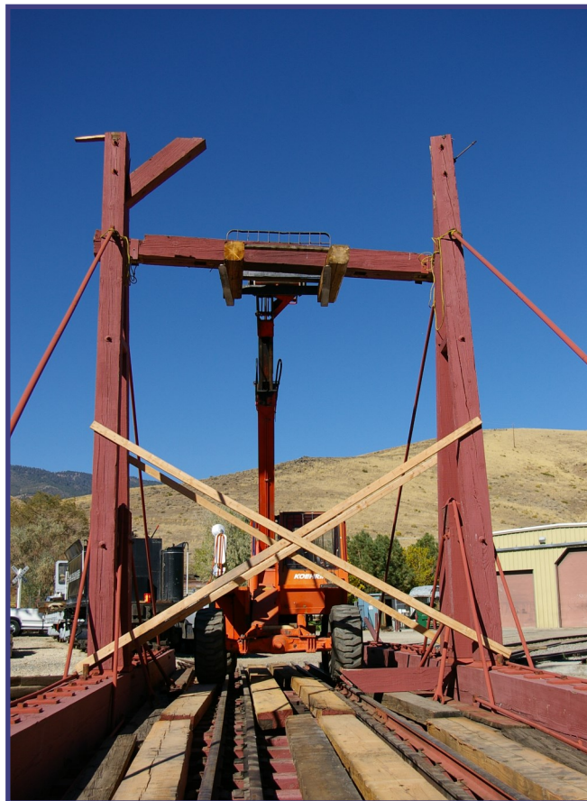
Shop staff remove the top sill of the A-frame after it became damaged in October 2014. (NSRM photo)
