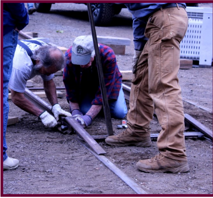
Laying the rails before building the ramp to take No. 5 off the trailer. (Photo by Cristol Digangi)
