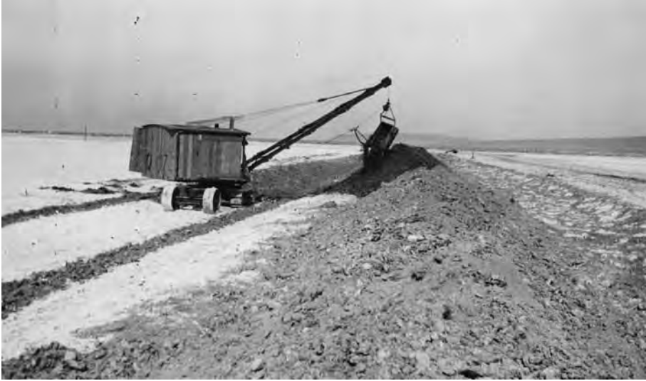
Figure 6: Road construction in Nevada, ca. 1920s. Photographer unknown. ( Lincoln Highway Digital Image Collection, Transportation History Collection, Special Collections Library, University of Michigan )
