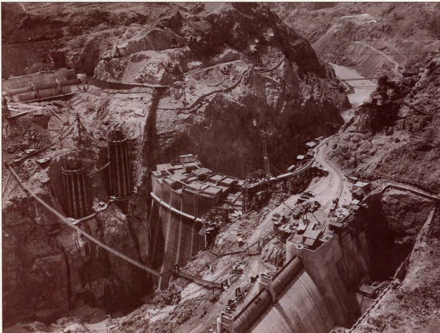
The intake towers rose from Black Canyon as the dam and spillways took shape. Lake Mead later formed on the left.
