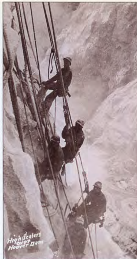
High scalars, in a dangerous job, prepared the canyon walls for blasting.
